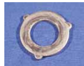
Washer showing evidence of substantial movement in the joint.
